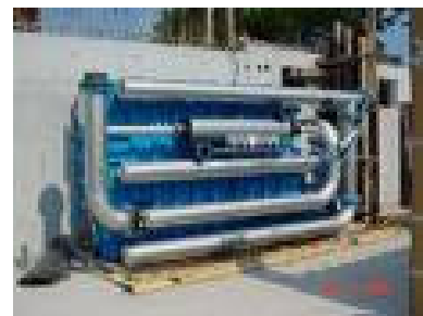
Swimming pool water treatment
